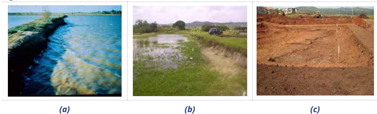
Figure 17: Erosion of Pond Walls
